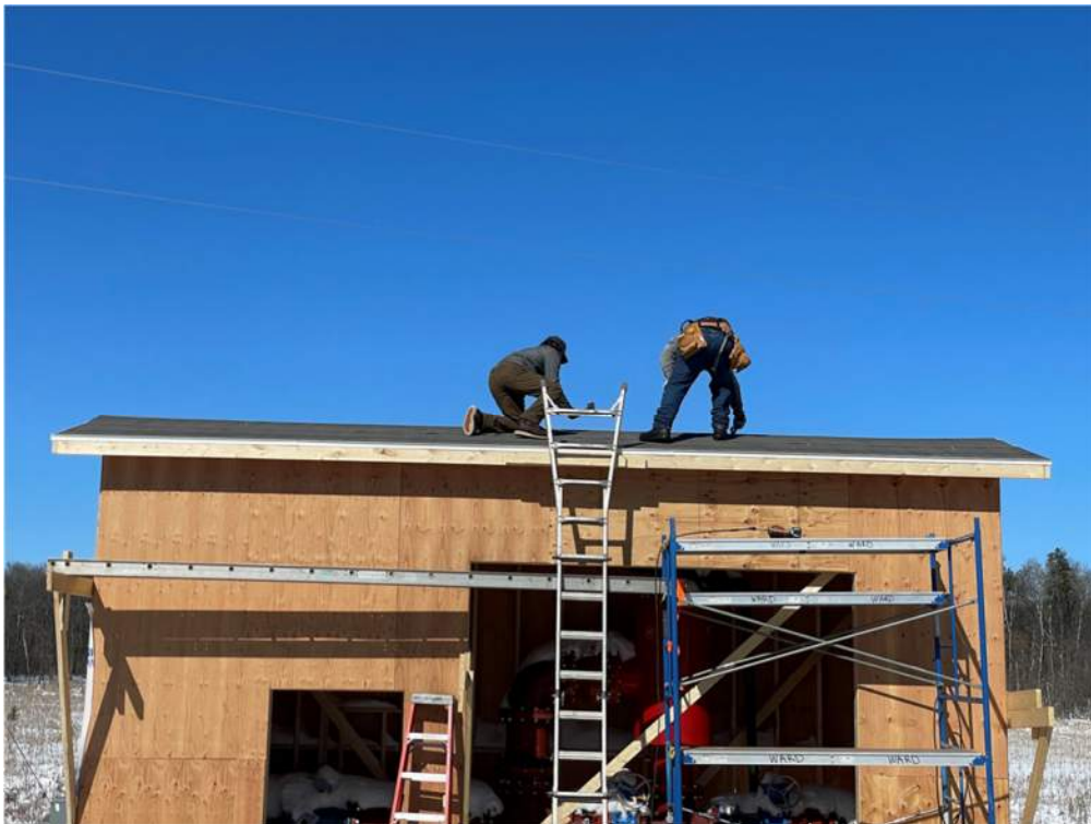
Photo #6: Installing underlayment before the shingles go on the roof - Mar 28, 2024, 11:00 AM
