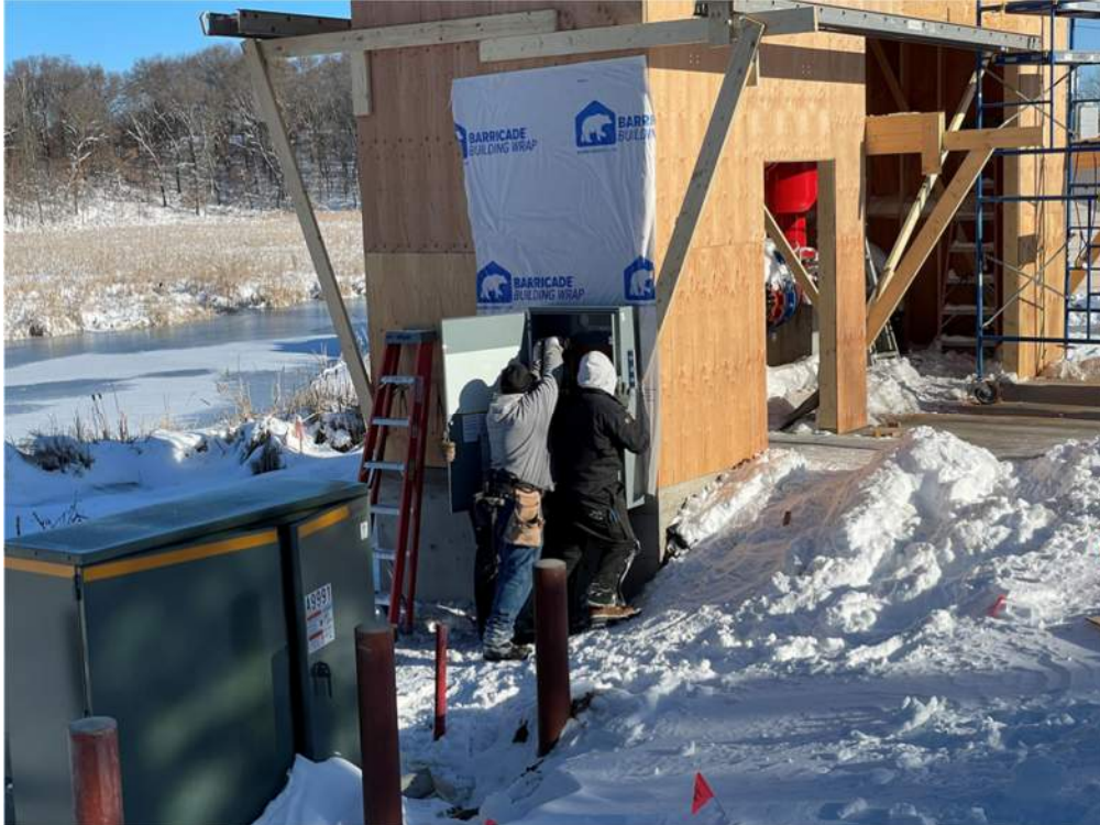
Photo #5: Design Electric is installing an electrical box on the outside of the pump house - Mar 28, 2024, 9:03 AM
