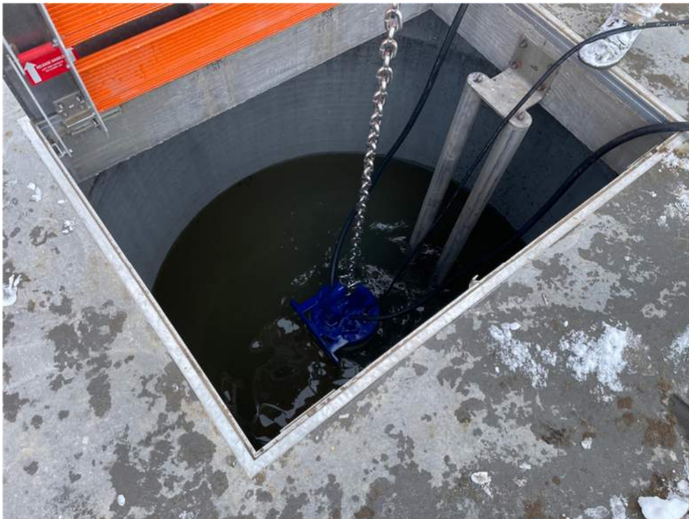
Photo #4: Pump lowered into wetwell and being guided down by the rails - Mar 27, 2024, 4:59 PM
