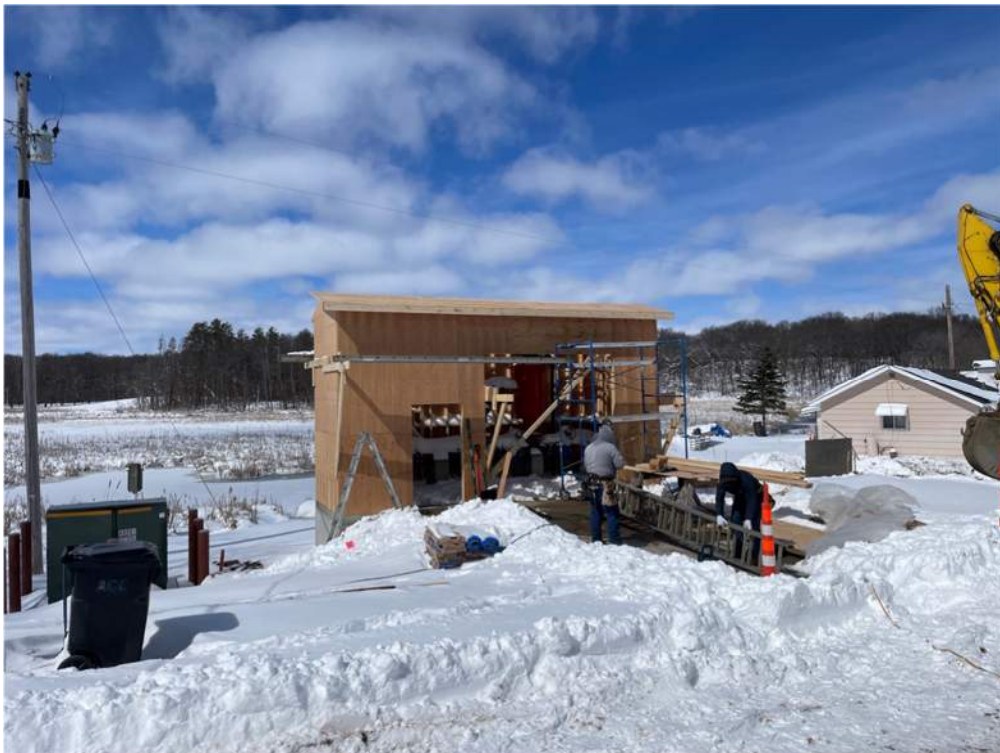
Photo #2: Plywood nailed onto the entire roof of the pump house - Mar 27, 2024, 1:19 PM
